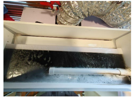
Figure 10. Upper Header Tank
