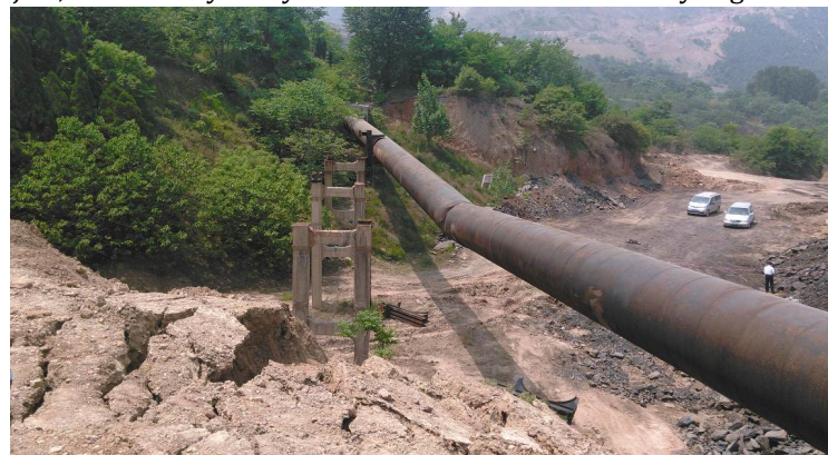
Figure 1. Damage to the aqueduct pipeline
