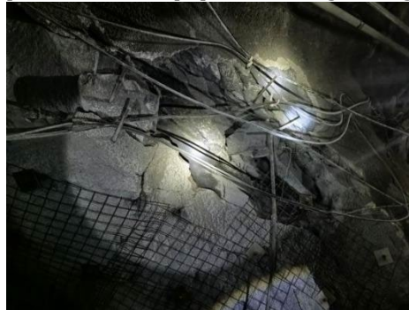
Figure 1. Local Concrete Roof Collapse and Spalling
