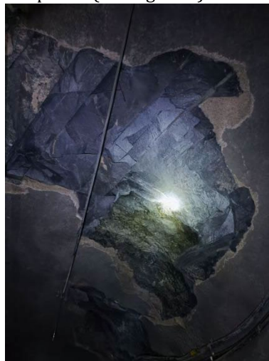
Figure 2. Concrete Spalling Caused by the Combined Action of Blasting Vibration and Rock Mass Stress
